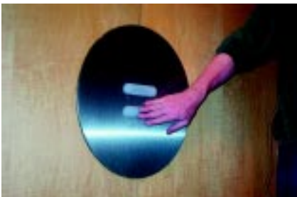
Figure 3. The absence of detectable information makes these elevator call buttons difficult for first time users with reduced vision to recognize.
